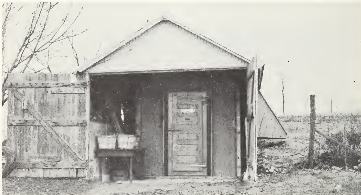
Figure 2.--Installation in a garage; compressors in lean-to.
